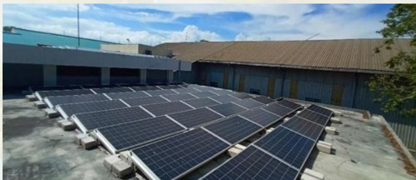
Gambar 42 Solar Panel di Atas Sub Station I BPG
