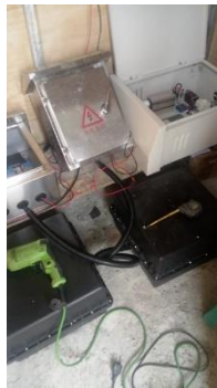
Gambar 2.8 Instalasi Solar Cell
