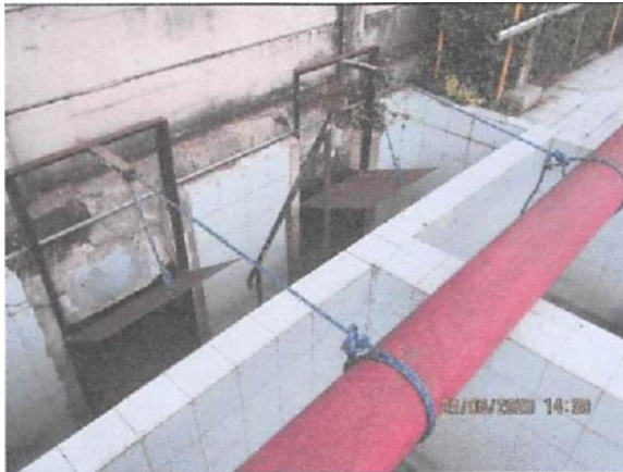
Gambar 4.4 Water Discharge Arranger Oil Catcher 2
