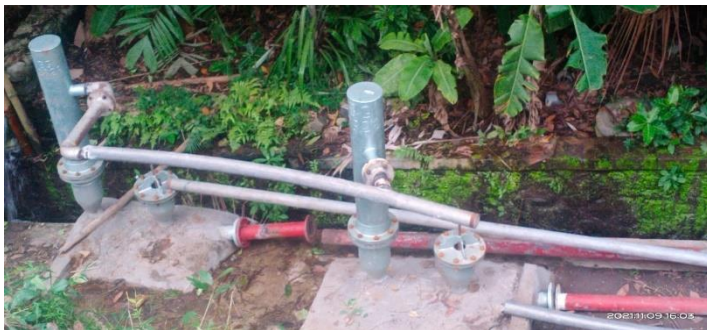
Gambar 1.2 Tampak Depan Pompa Hidram “ Green Hydrant ”
